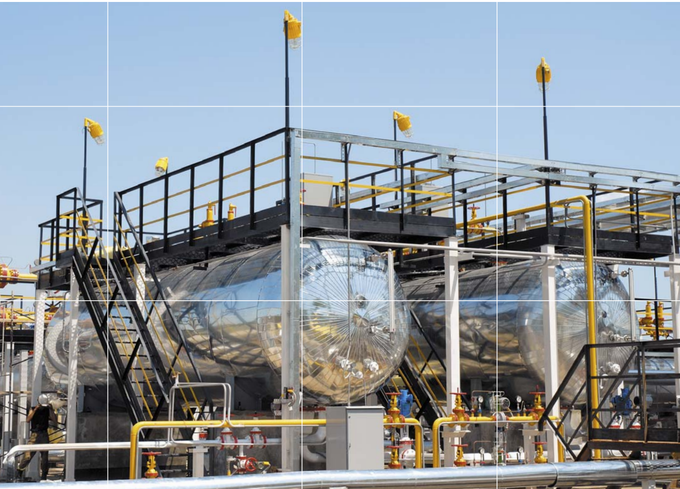
Separator (part of oil&gas group installation №58) at LLC RN-Krasnodarneftegaz
