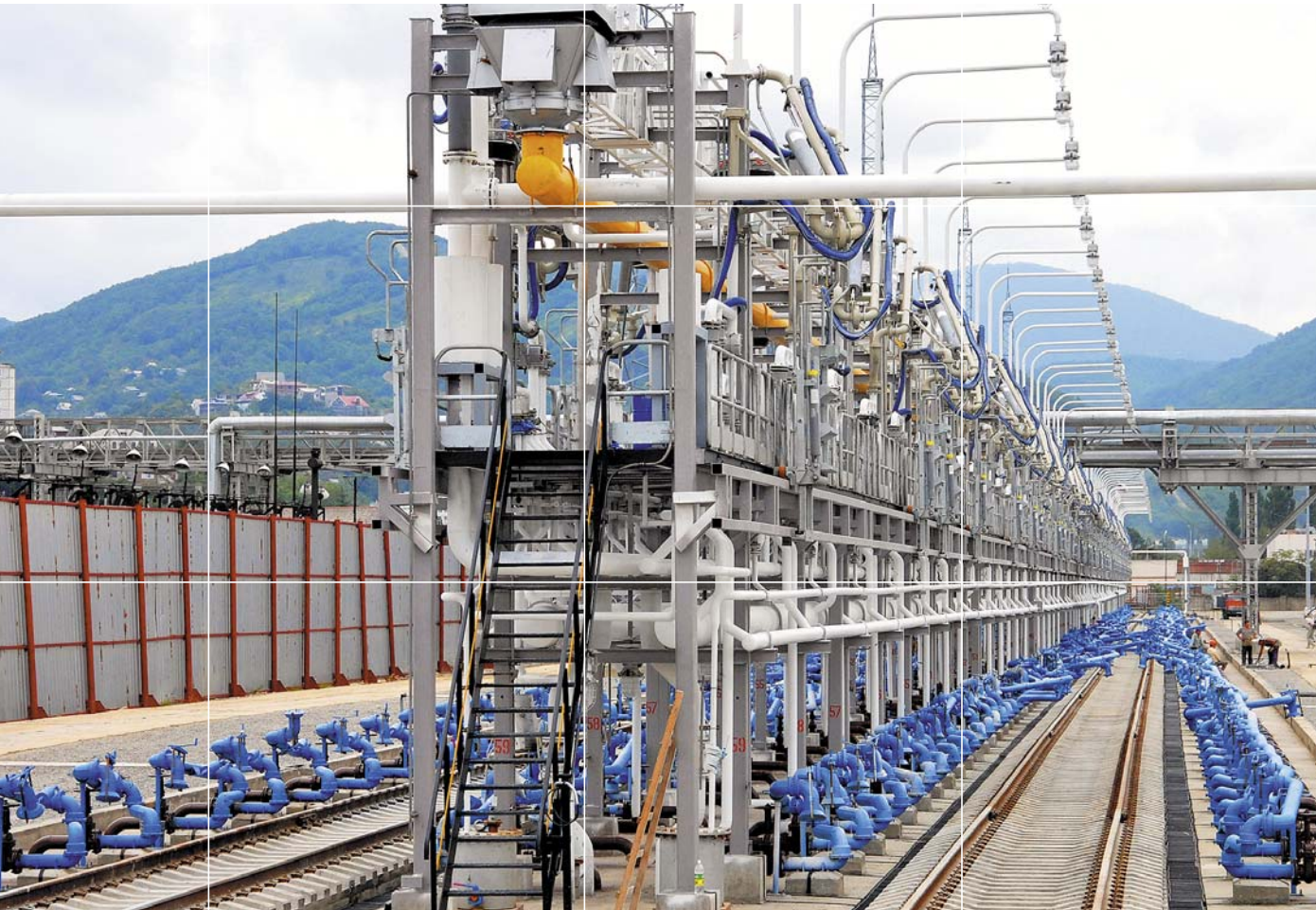
Oil loading rack at LLC RN-Tuapsenfteprodukt
