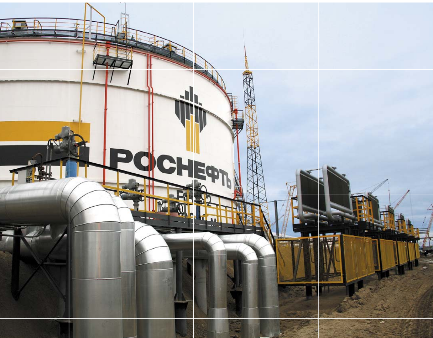
Water discharge unit at Vankor
