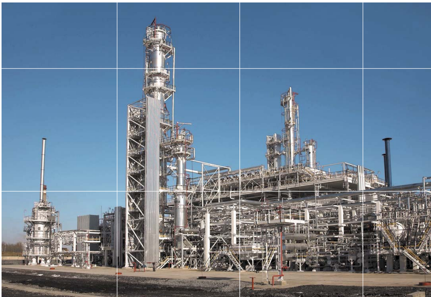
Isomerisation unit at the Achinsk refinery
