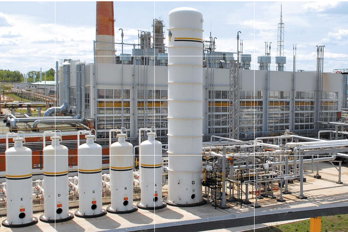
Short-cycle adsorption unit at the Novokuibyshevsk refinery
