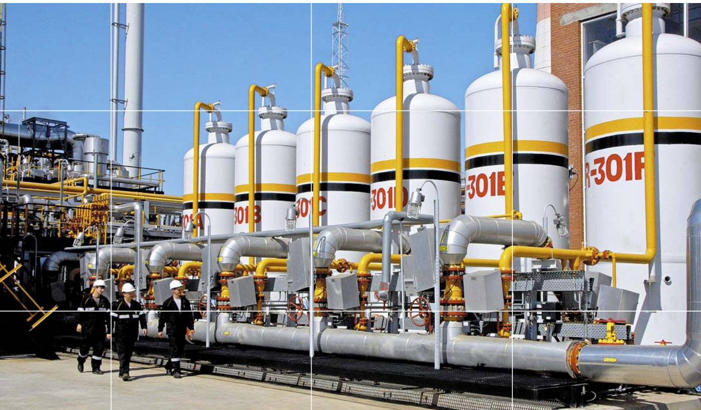
Hydrogen production unit at the Kuibyshev refinery
